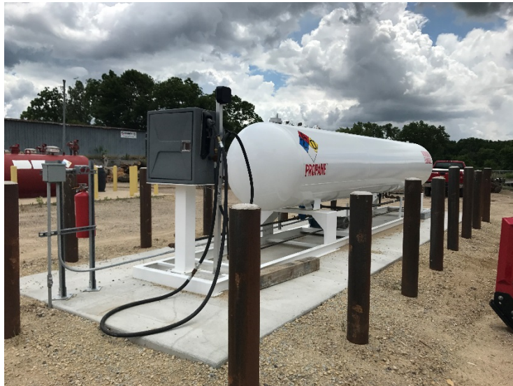
On-Road Propane Fueling Station-2000gal
