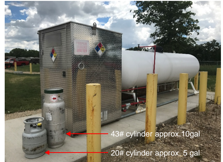
Off-Road Equipment Propane Fueling Station-1000 gal
