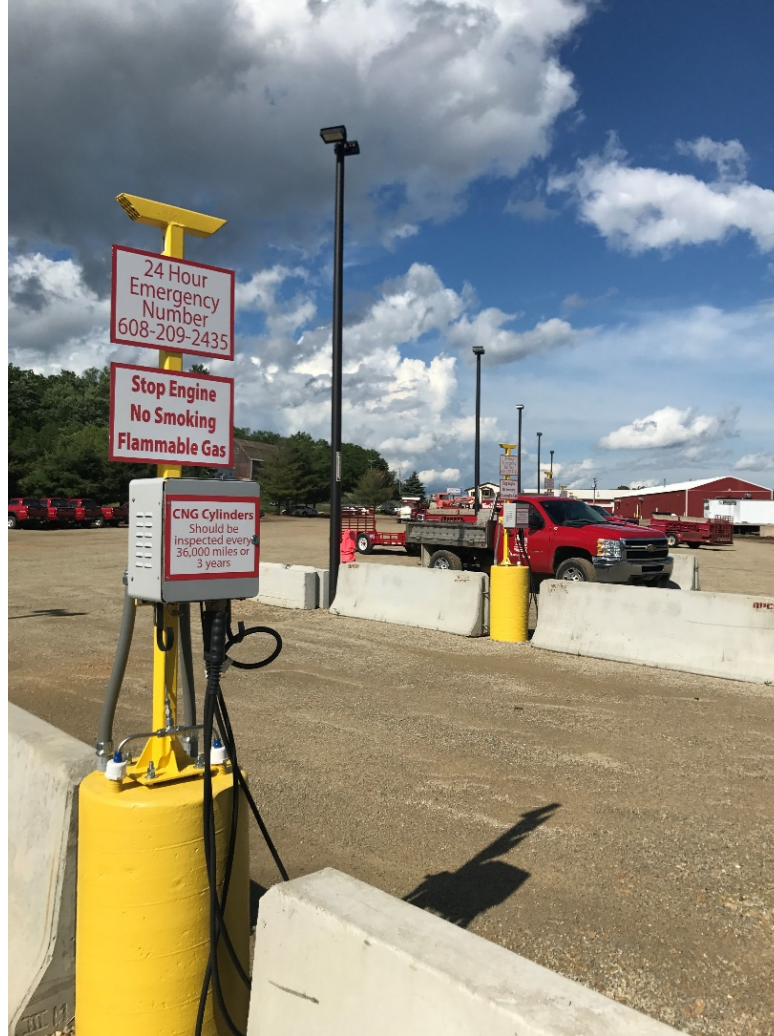
Dual Fuel Posts
